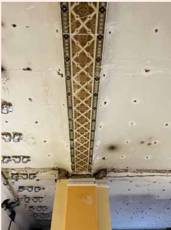
When they opened up the ceiling of the Garden Hall, the building team revealed decorative features from the past.
